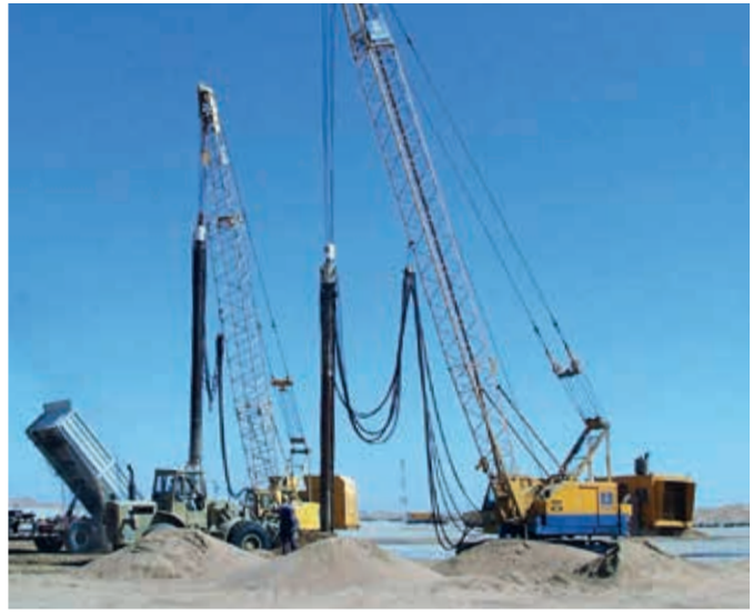
Crane with power pack
